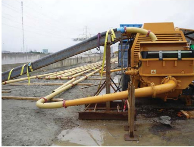
Figure 1: Layout of the closed-loop pumping circuit with a total length of 600 m
