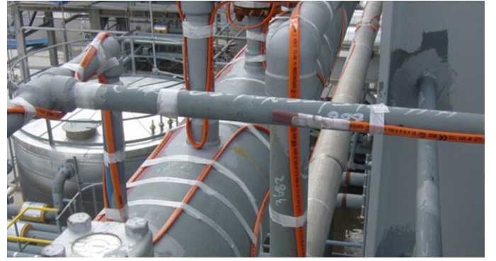
Fig. 4. Industry example of heat tracing placed on pipes [10].
