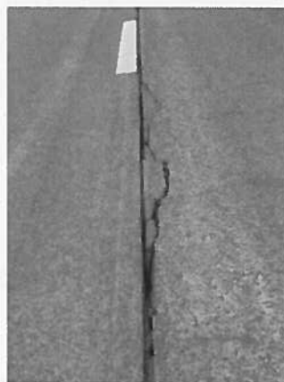
Figure 2. Widening of the longitudinal joint and cracking over a width of 100 to 150 mm along the joint
