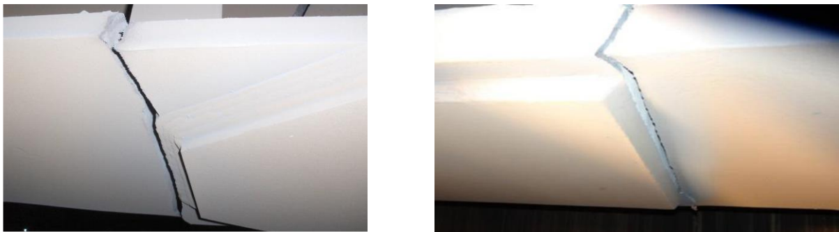
FIGURE 6: Fatigue cracks observed at cover plate ends in the bottom flange of crane girders
